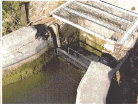
5 - Culvert from the lake to the New River tributary west of project site
